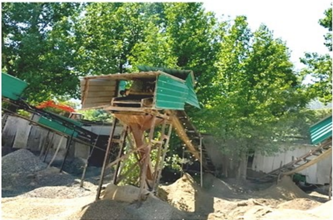
Photograph 04 (g & h): Covering of Conveyor belt and Material transfer point with sprinklers
